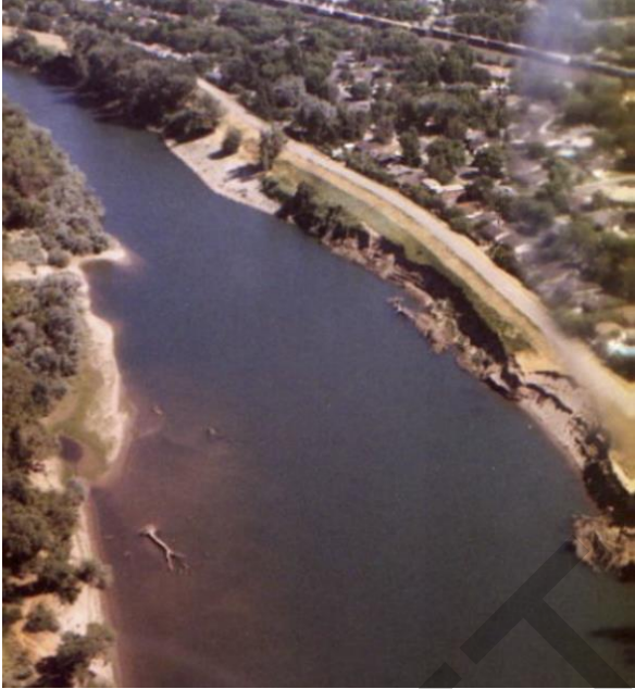
Figure 9-2. Erosion Below Levee Toe in Foundation (USACE Sacramento District).
