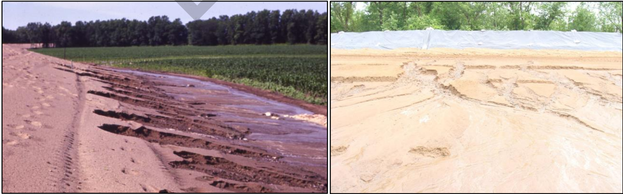
Figure 0-14. Sloughing Due to Seepage through Steep Sand Levee Sections. Photos courtesy of USACE Rock Island District.
